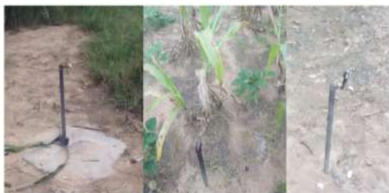
Plate 4: Only two out of 5 water faucets in Gurungu and Sharifai are functional
