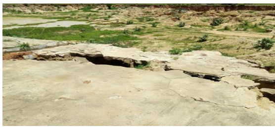
Figure 7: Eroded Barricade Constructed to Avert Road Encroachment from a Neighboring pit Source: Field Survey, 2026
