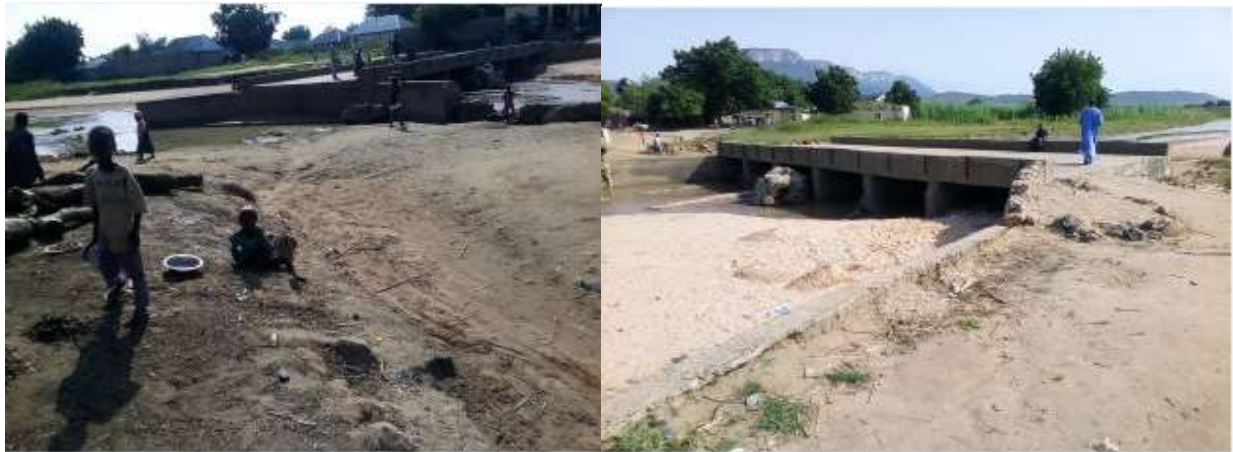
Figure 6b: Damaged Gada Dauda during the 2017 Dadin Kowa flood
