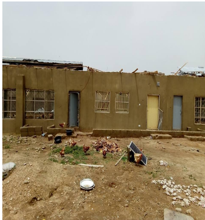
Plate 2: Poultry house damaged by wind at study site Source: Field Survey, 2019.
