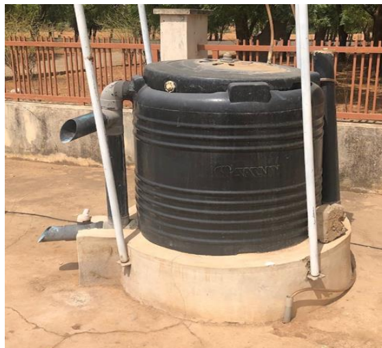
Figure 1: Floating Dome digester
