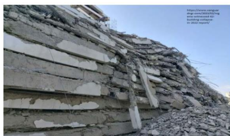
Figure 1a: Typical collapsed building (Source: Vanguard News 2024)
