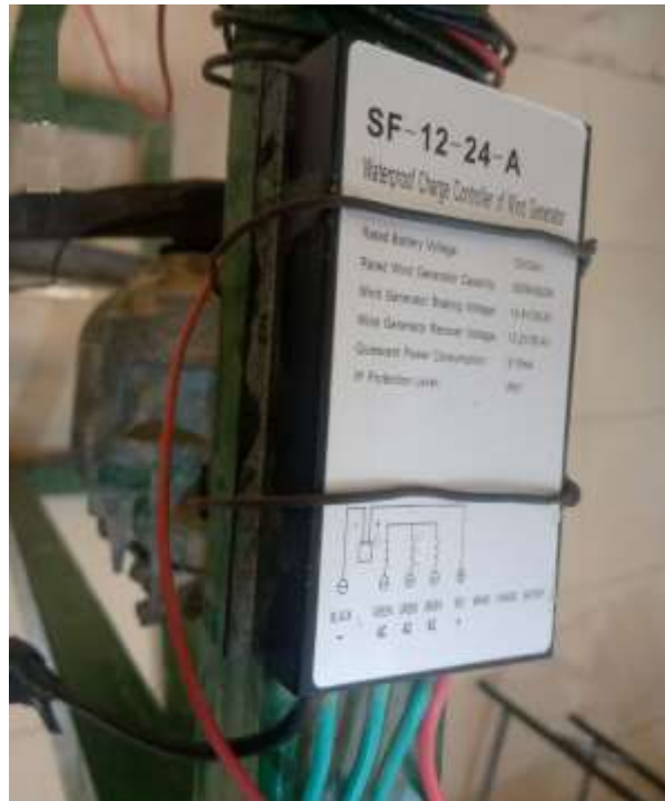
Figure 4. The wind turbine charge regulator
