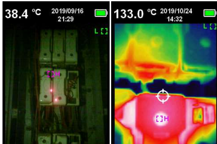
Figure: 4 (a) three-phase distribution board, (b) thermal image of the main distribution board
