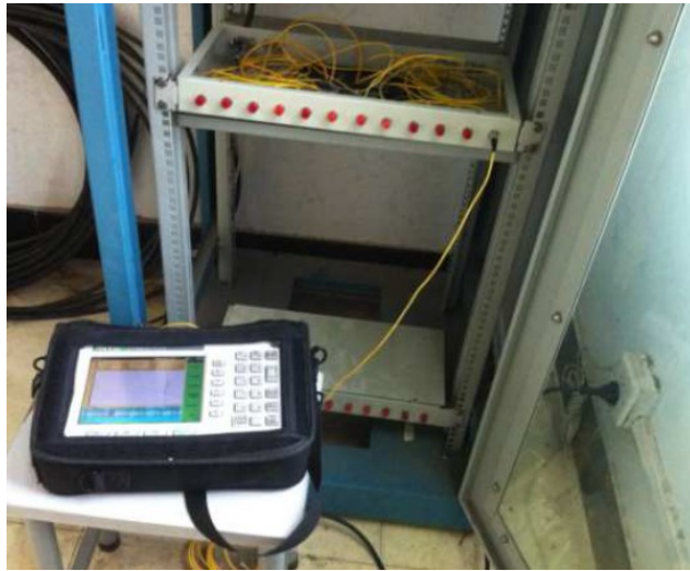
Figure 1: OTDR connected to fiber under test
